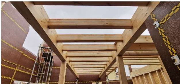
Fig 16. Pilot house of the LIFE Wood for Future project incorporating laminated poplar wood beams from the Vega of Granada
